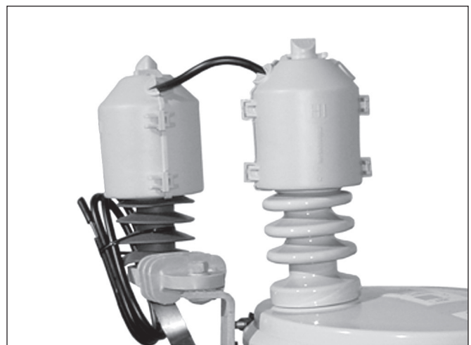
Figure 1: 2140 Wildlife Protectors installed on overhead distribution transformers.
